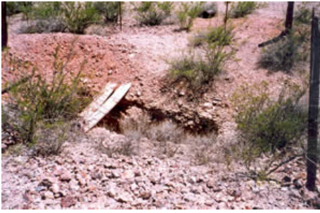
Opening to flourspar mine. The cavity was 42 ft deep immediately underneath and connected to other openings in the area.
