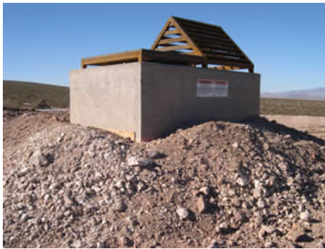
A new concrete support wall was placed around the old one. A cupola for bat passage was placed on top. The flat portion is covered with steel grating that can be removed for entry by bat biologists.
