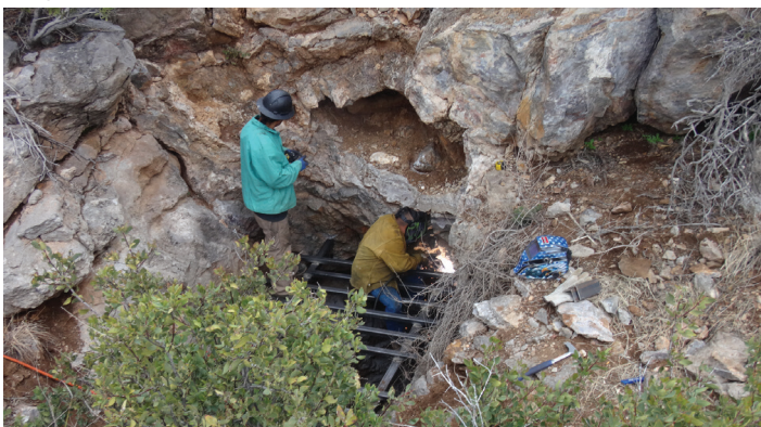
A bat gate being constructed over a mine shaft at the Cookes Peak East Mine Safeguard Project – Phase II.
