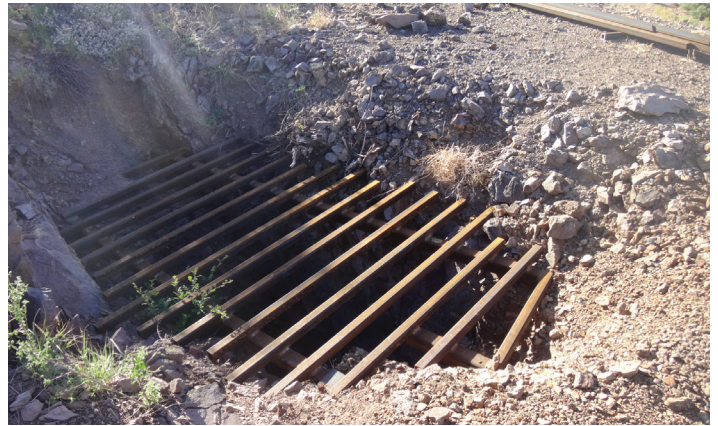
A finished bat gate constructed over a mine shaft at the Cookes Peak East Mine Safeguard Project – Phase II. The gate will allow birds and bats to come and go while safeguarding humans from a vertical drop.
