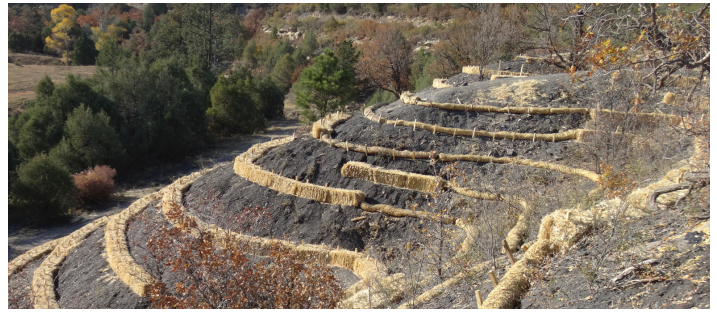
Constructed terraces with straw bale at the Tin Pan Canyon Reclamation Project will slow the water runoff and support newly planted seedlings.
