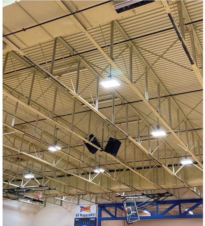
Socorro High School Gymnasium LED Lighting Upgrade (Socorro Consolidated School District ESPC project)
