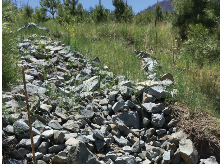
Zuni Bowl construction and associated fishbone style berm to remediate headcut and downhill erosion, 2020
