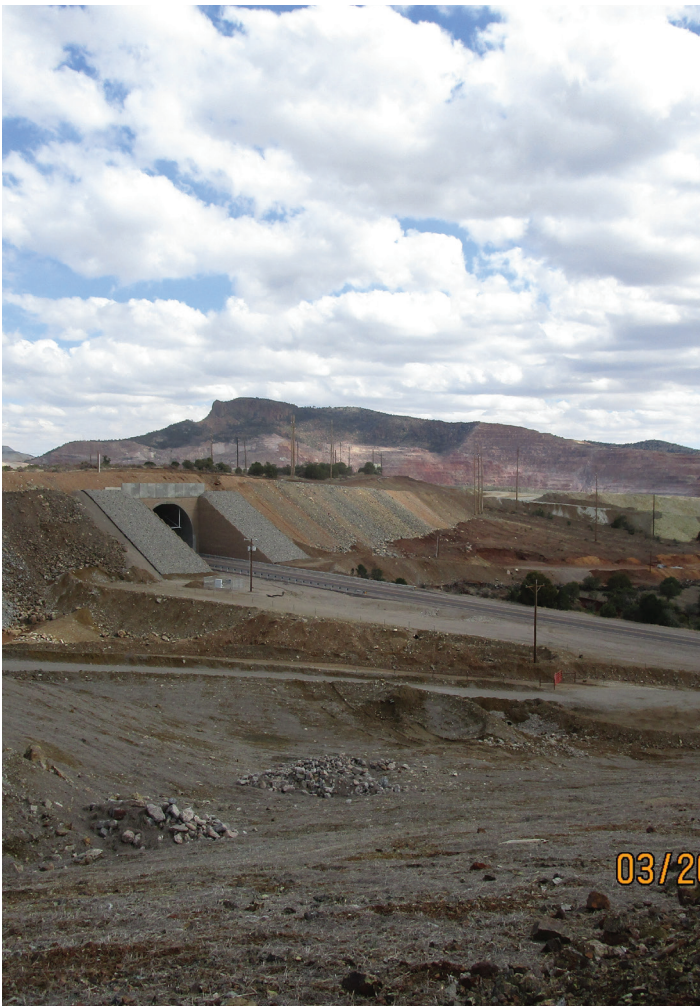
Main haul road between Continental and Chino, showing bridge and Overlook Tunnel across State Hwy 152, Continental Mine, Grant County (2019)
