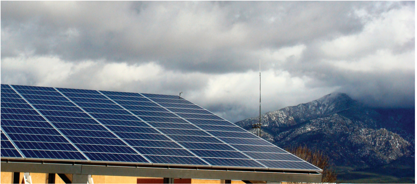
Solar panels at Taos High School
