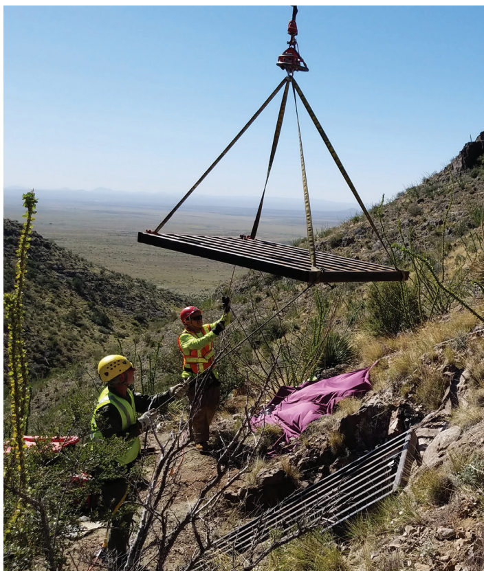
Helicopter delivery of a prefabricated steel mine gate on steep, rugged terrain at the Cookes Peak West Mine Safeguard Project – Phase IIIB.
