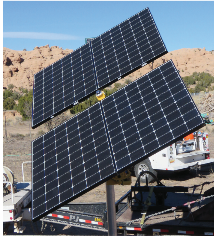
PV on a Pole installation on Nambe Pueblo.
