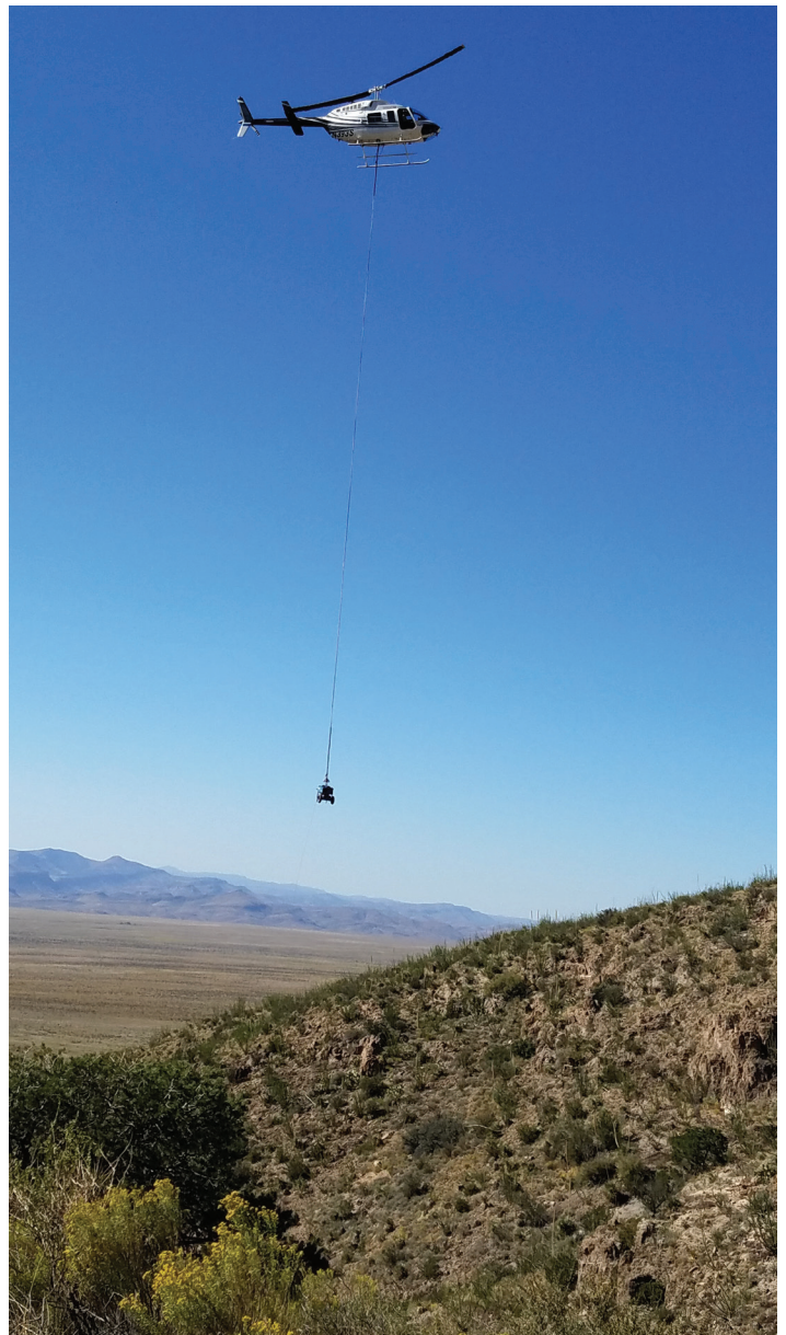
A helicopter delivering a steel bat gate to remote location at the Cookes Peak West Mine Safeguard Project – Phase IIIB.
