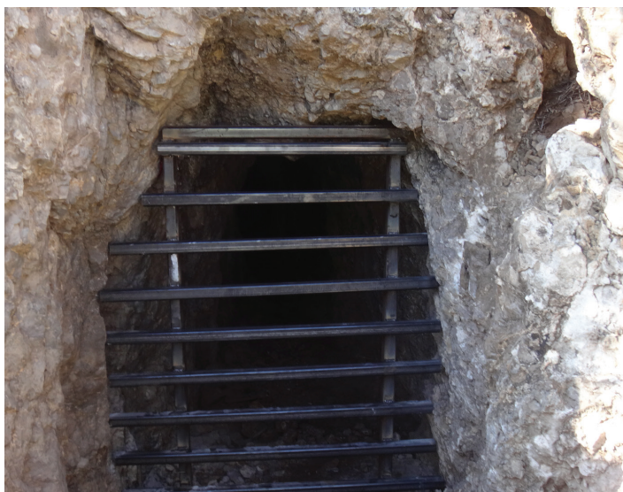
Steel bat gate constructed in place at a mine adit as part of the Cookes Peak West Mine Safeguard Project – Phase IIIB.
