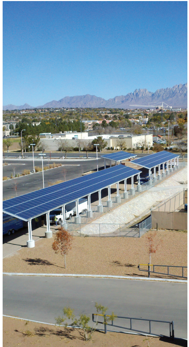
Solar installation on the Las Cruces Convention Center
