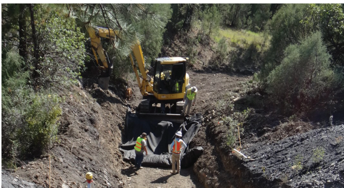
An eroded drainage channel through a coal waste pile being constructed into an engineered rock rundown at the Tin Pan Canyon Reclamation Project.
