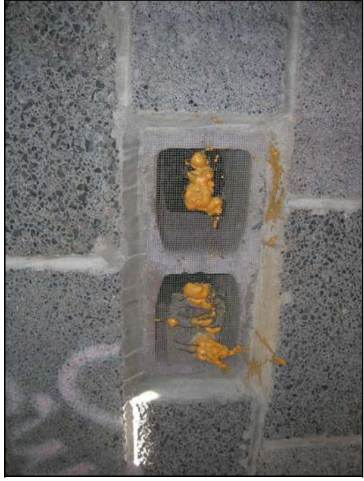
Screened in vents as a precaution against embers, Sherwood Forest residence. Source: Sam Amato, USFS
