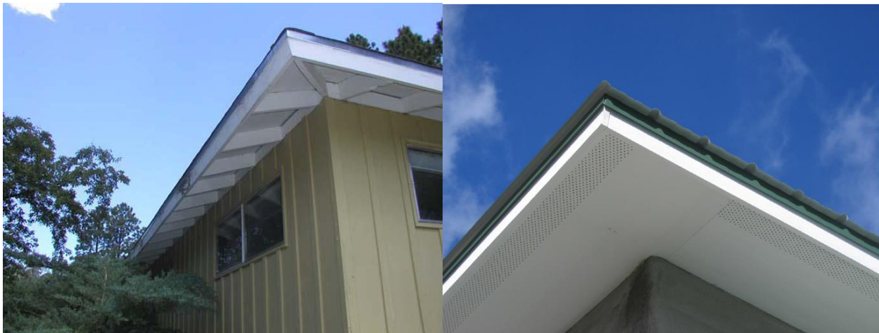
Rather than exposed eaves, the current interface code requires new construction to include eave protection from firebrands.
