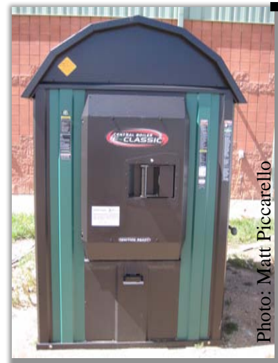
Image 3. Cordwood boiler installed outside of transfer station
