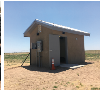
New blower building serves to aerate the septic tanks for odor control at Oasis.
