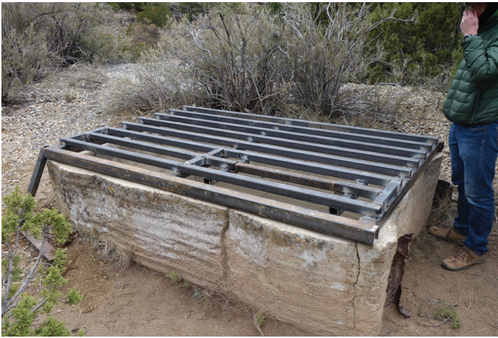
A safety closure at the San Pedro Phase II Project constructed over an old mine shaft collar by the BLM's contractor
