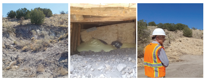
Pre-construction conditions at Bethlehem Hill in Madrid Foam "bag bombs" were tossed into this reopened adit and punctured with a long pole to plug the sides of the backform and prevent foam drainage deeper into the adit Former AMLP Manager, John Kretzmann, observing the completed Bethlehem Hill Project with the contractor
