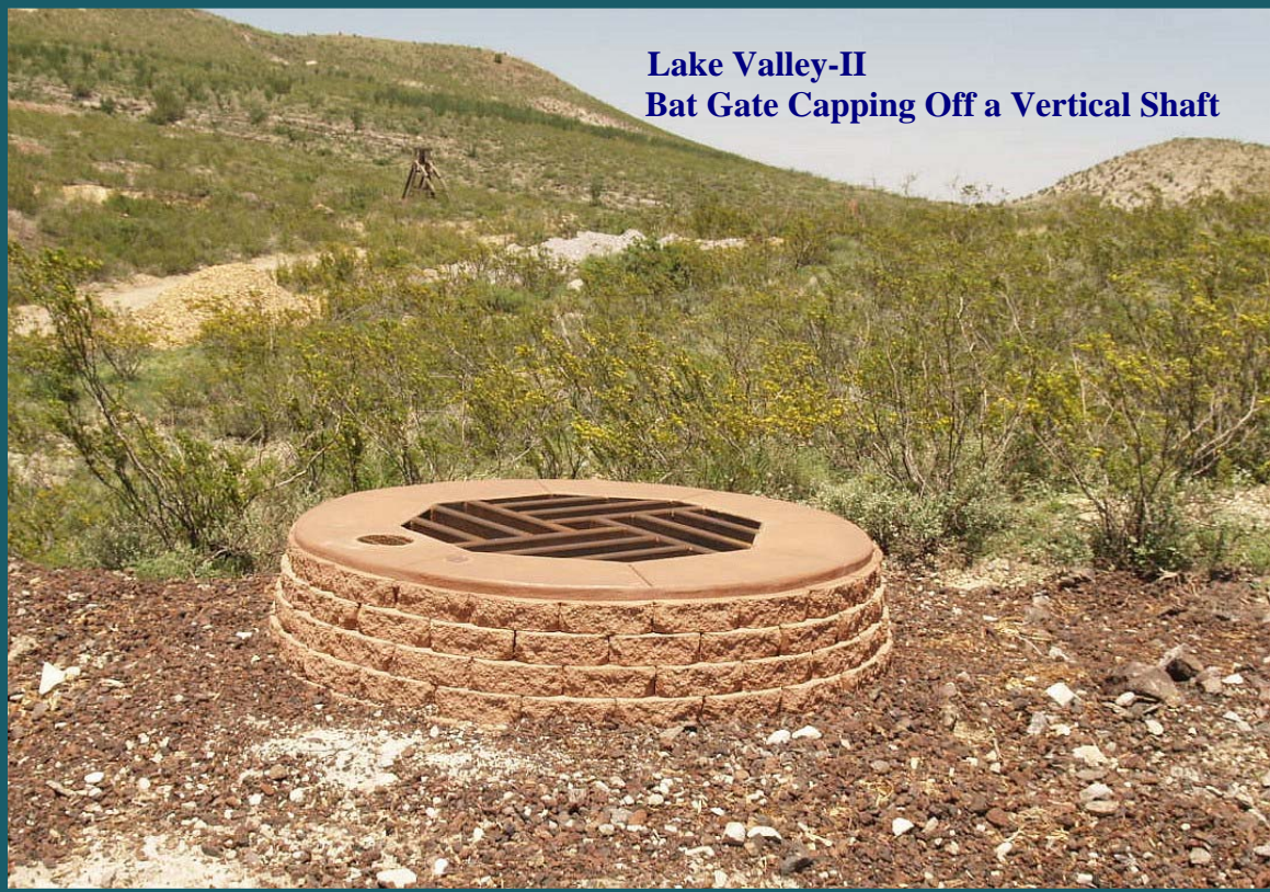
Lloyd Moiola, Inspecting Installation of Corrugated Metal Culvert. Culvert Is Placed into Mine Drift to Protect the Integrity of Underground Workings and to Accommodate Bat Access and Airflow.
