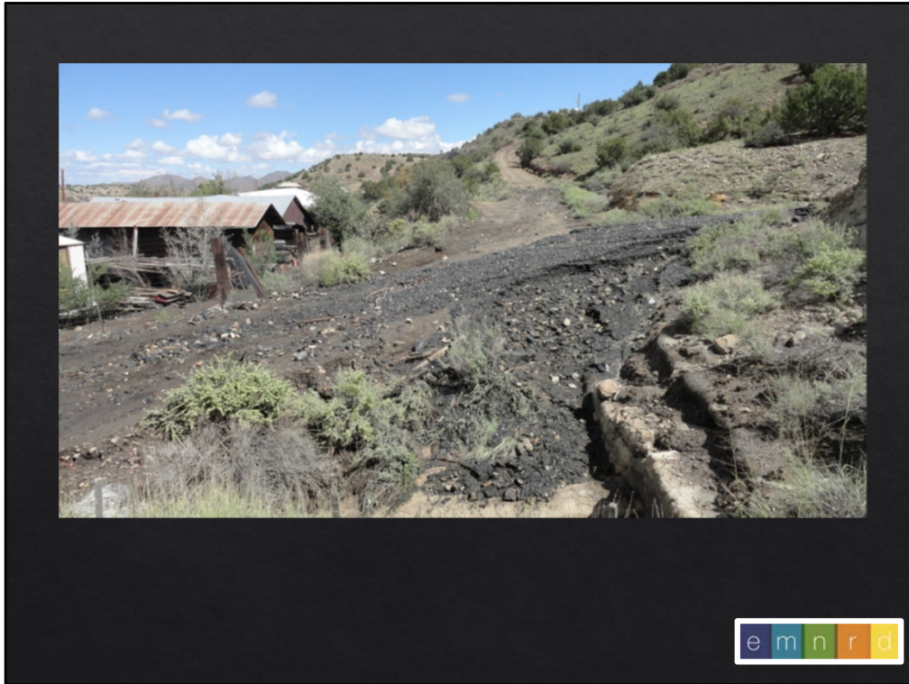
This shows the debris flow from a gob blowout across the driveway and onto Museum property.
