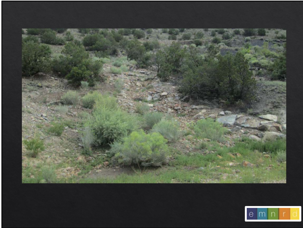
The completed step-pool rock bypass channel in August 2016. Note planted and seeded vegetation in and around the channel. The large light colored rock was covered with smaller tan rock to better blend channels into the surroundings.
